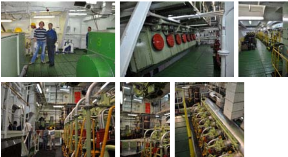
On Thursday we are allowed to visit the machine room.
