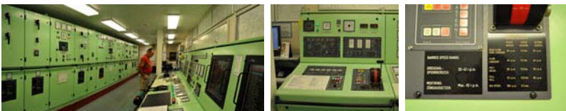
The control room; Main engine control.
