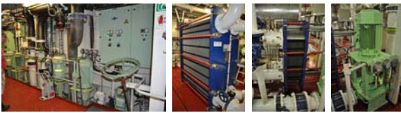
Main engine cooling: The sea-water pump pumps 450 m 3 /h salt-water at 1.6 bar to the heat exchanger and the fresh-water pump pumps 180 m 3 /h at 3 bar through the motor.
