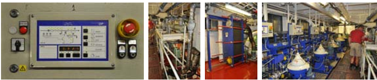
Lubrication oil heating, cooling, filtering.
