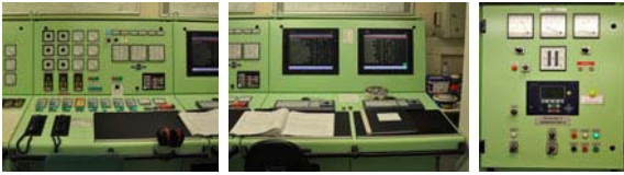
Alarm panel; Main parameter control and adjustment panel; Power generator control (1 of 3).
