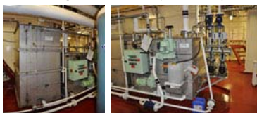
The biological sewage treatment plant can process up to 7.4 m 3 of black-water per day. The tank itself holds 2'000 l (2 m 3 ). Vacuum toilets like the ones known on plains are used on board to minimise the amount of water to be treated.
