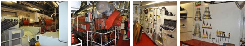
Three power generators driven by MAK diesel engines; Special tools and workshop for generator maintenance and repair.
