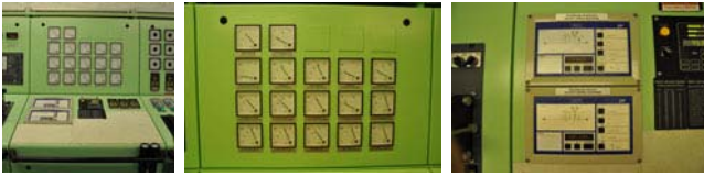
Viscosity control of lubrication oil; Pressure and temperature control of fuel, lubrication oil and compressed air.
