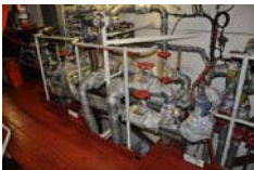
Fuel pre-heater for the diesel engines of the power generators.
