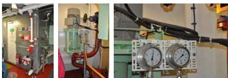
Fire hydrant water pump and vacuum/pressure gauges.
