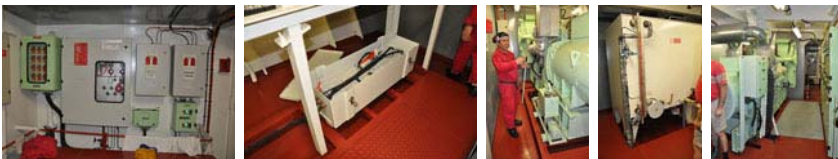
Emergency power generator. It is a completely independent system, has its own diesel tank and can be started by battery or even man power.
