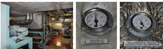
Air condition unit; Intake temperature; Output temperature
