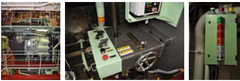
Main engine lower 2 floors: Emergency motor control panel; Common alert panel.
