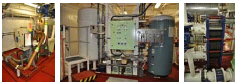
Fresh-water generator. The evaporator can produce 22 m 3 in 24 hours. The boiler is driven by main engine coolant.
