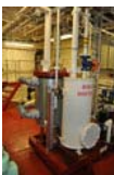
HFO fuel must be preheated before it can be burned. The heater heats up to 11.9 m 3 HFO per hour. Since the HFO is heated with the engines coolant, the main motor must be operated with standard diesel fuel until the HFO reaches the right temperature.
